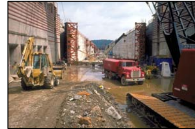
Repair Plans and Costs
